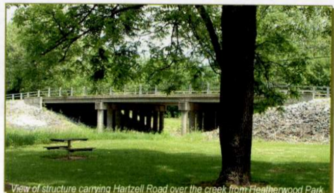
View of structure carrying Hartzell Road over the creek from Heatherwood Park.
